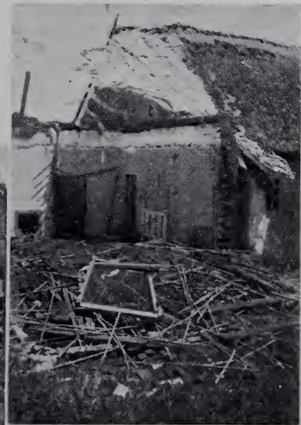
The room in which Mr. Lees and the others were killed. Photographed after removal of most of the wreckage.
